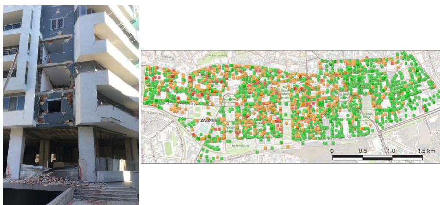
Fig. 2 a Damage and collapse of infill walls in a 2-storey RC building in Durrës during Albania earthquake (MW 6.4) of November 26, 2019 [18] and b building usability in the Lower town of Zagreb after the M_w 5.4 Zagreb (Croatia) earthquake of March 22, 2020 [1]
